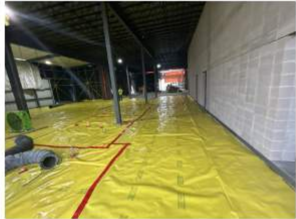
Vapor barrier installed ready for wire mesh and concrete. Looking North down corridor by locker rooms
