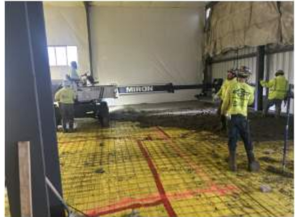
1 st concrete pour on the turf room. Laser screed was used to get the perfect flatness
