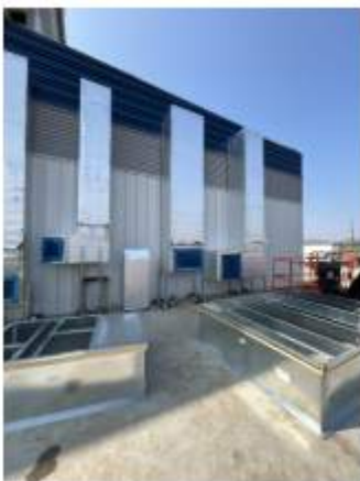
Northwest ductwork installed
